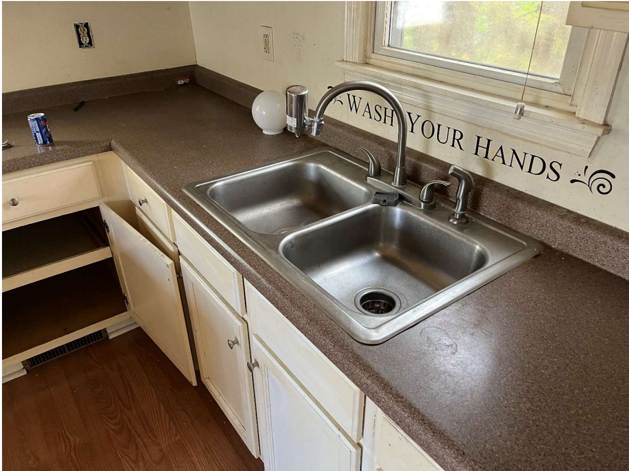
Photo #1 – Kitchen. Sink with asbestos containing undercoating.
