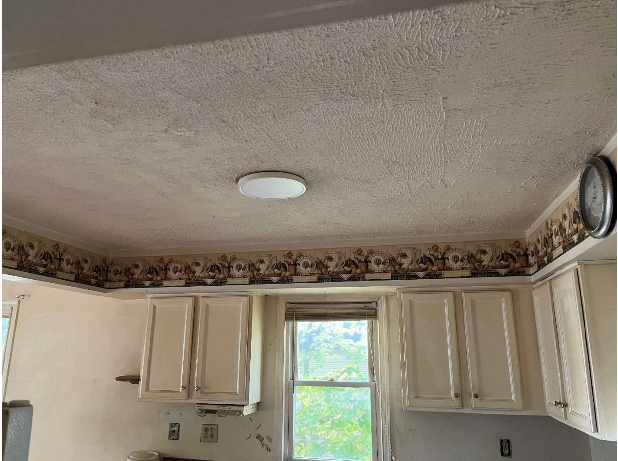
Photo #2 – Kitchen. Ceiling texture found to asbestos containing.
