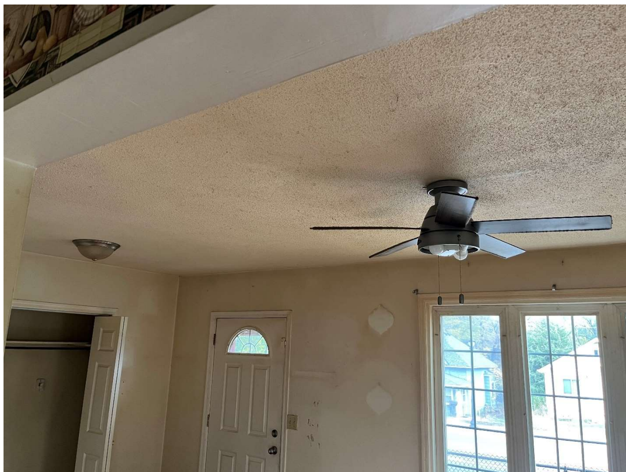
Photo #3 – Living Room. Asbestos containing ceiling texture.
