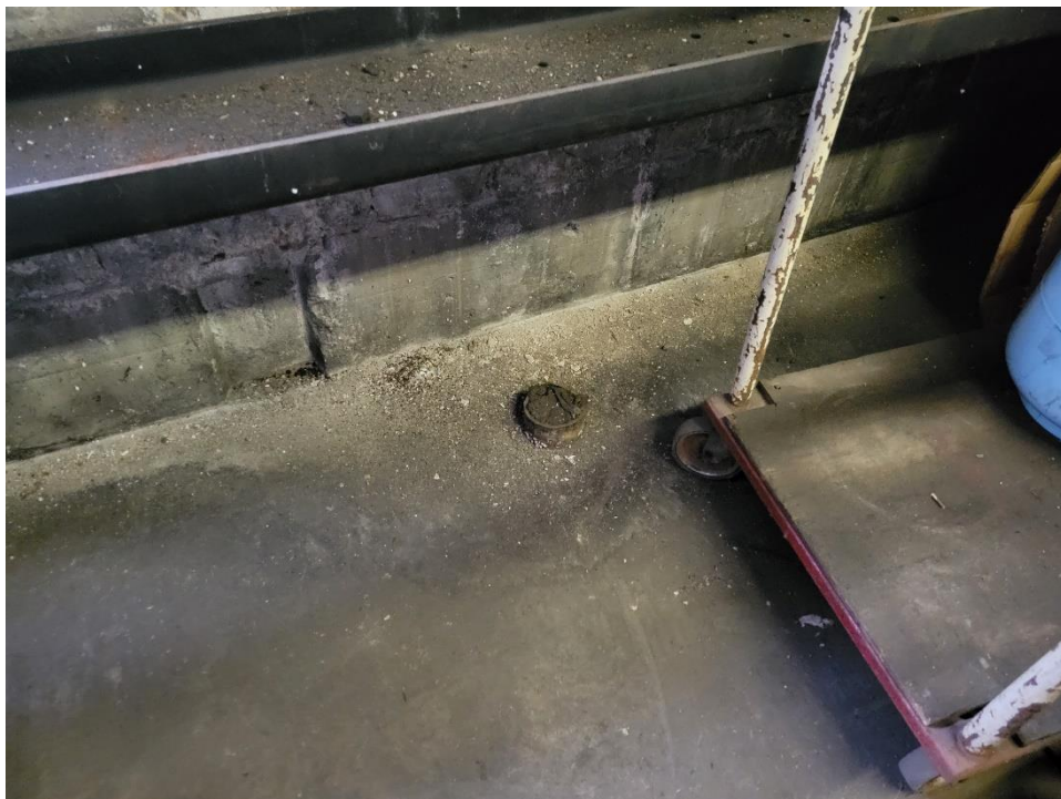
A hollow pipe in the floor of room adjacent to old garage.
