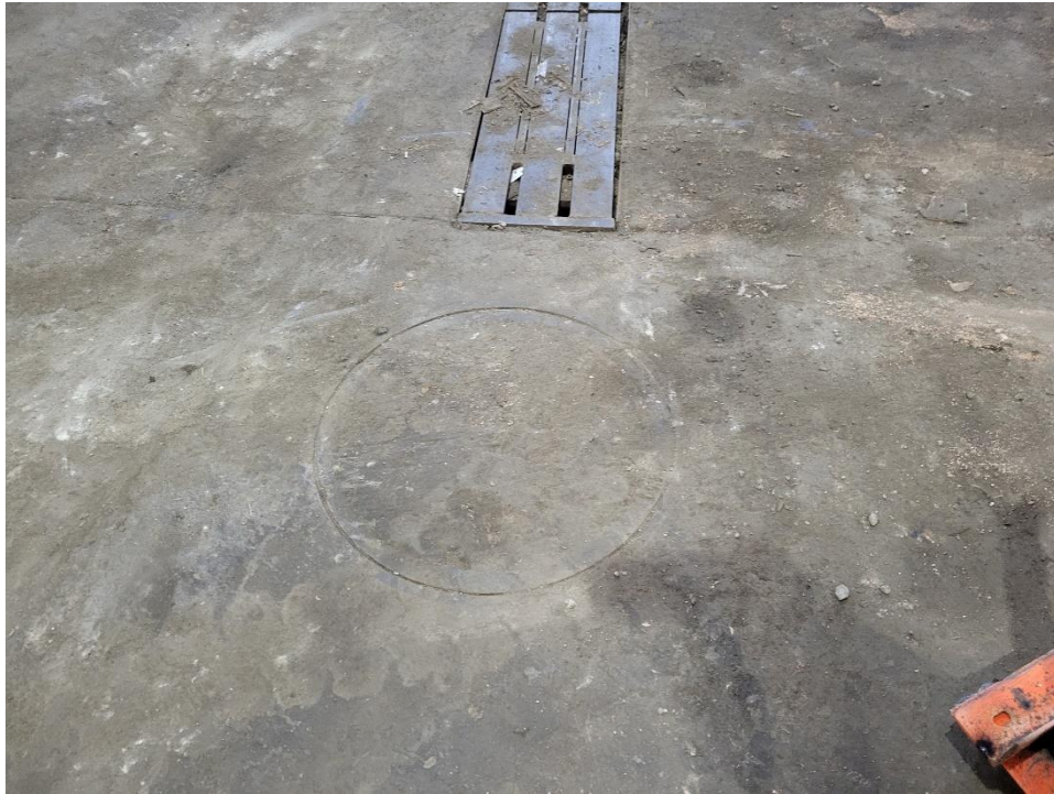
Oil water separator in newer garage.
