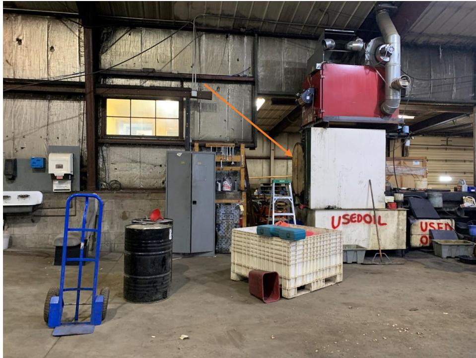
Used oil furnace and 400-gallon AST in newer garage.
